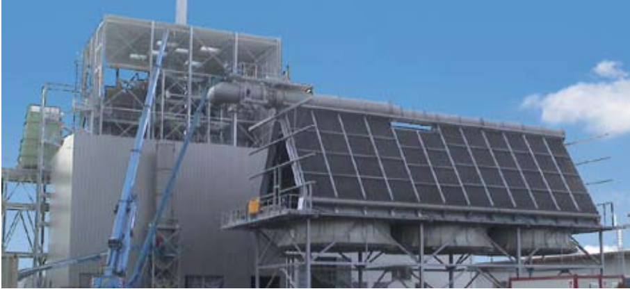
The Heiligenkreuz Biomass Plant, Austria is installed with Clyde Bergemann TERMOTEC air condensers
